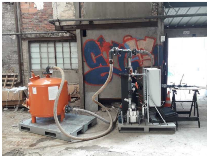
Figure 14 : Skid de venting
