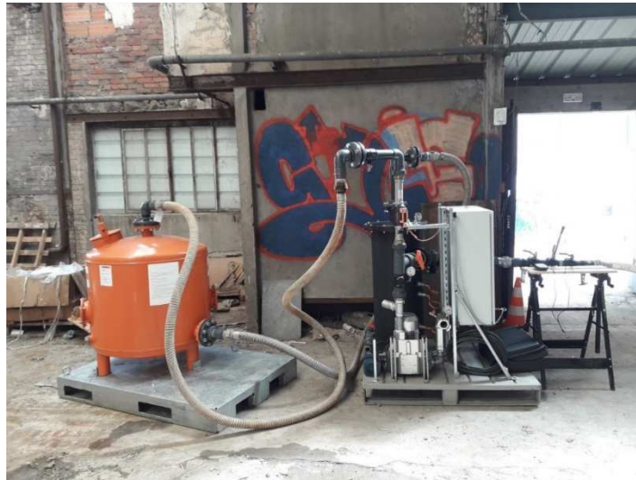
Figure 3 : Skid de venting
